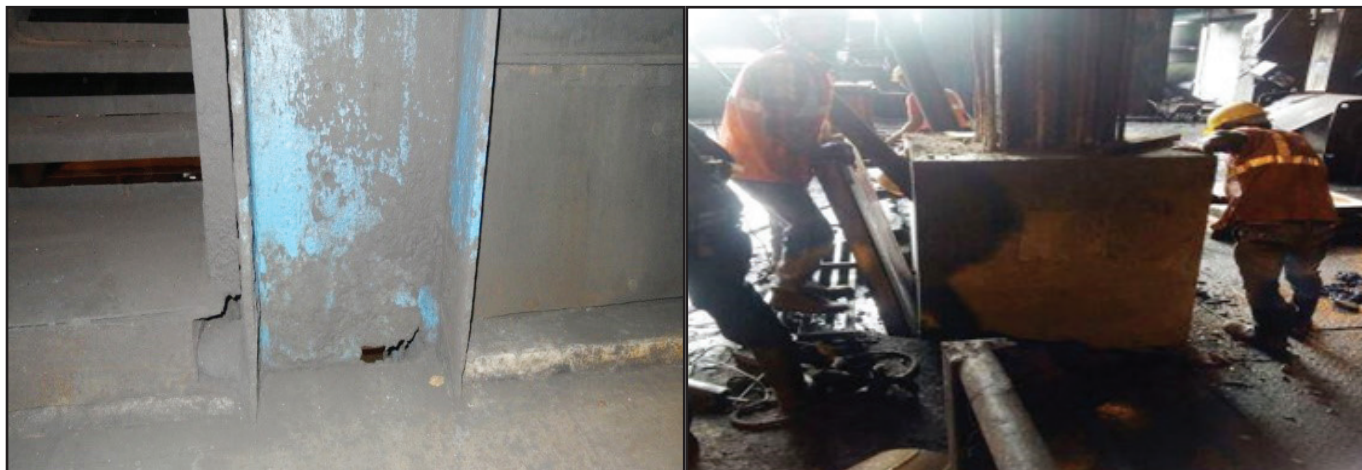
Figure 1A & B – Web of column corroded away & concrete augmentation
