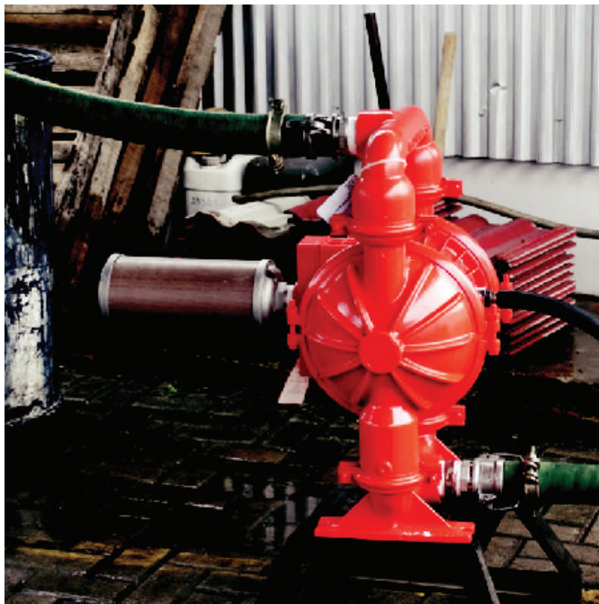
Installing the revolutionary PRO-FLO-SHIFT ADS on a Wilden Bolted Series AODD Pump for its solvent handling operations
