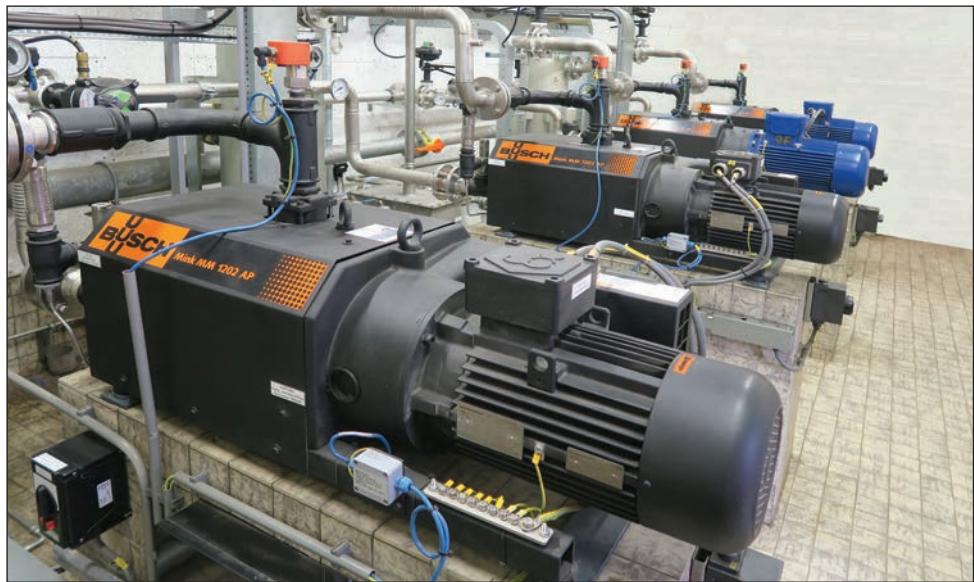
Figure 3: Compression and thus transport of biogas by means of four Busch MINK compressors. ©Busch Dienste GmbH
